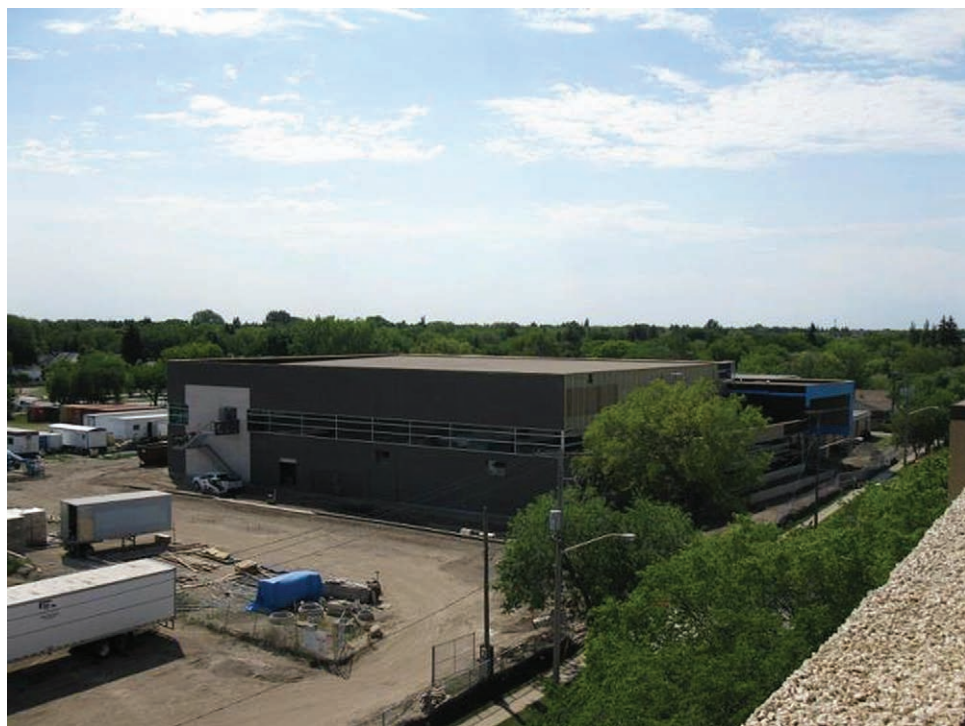
The new Healthy Living Centre as on August 10, 2012, in construction as of printing. Article on page 3. Photo credit http://www.brandonu.ca .
